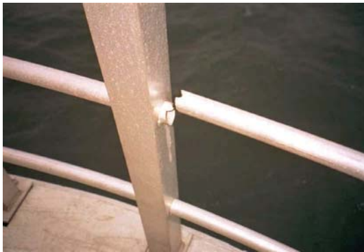
Figure 8: The distance between the posts in the fence has been too large creating vibrations caused by the wind. The repair is simple.
