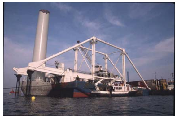
Figure 14: The floating crane with a foundation and the lower part of the tower at the site just before placing
