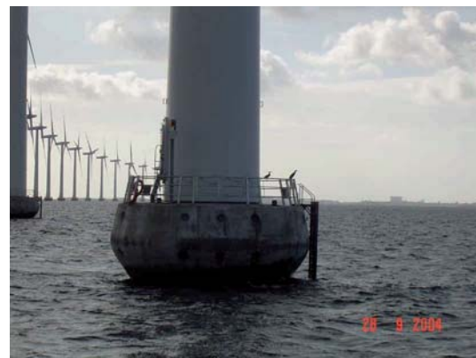
Figure 9: The access ladders for smaller boats are damaged after winters with ice. A special weak link is build into the ladder in order to limit the damage.
