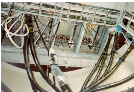
Figure 11: Cracks have developed, where the cables are entering the switchgear
