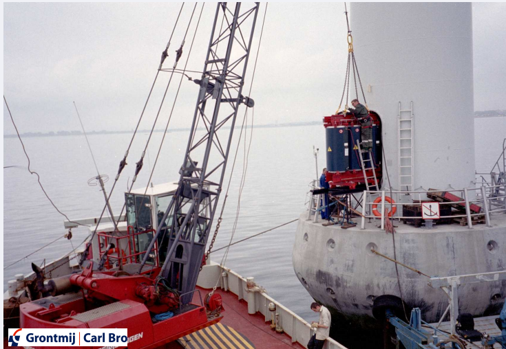
Fig. 1 Installation of transformer by working vessels. The space is very limited in the tower and there is only 1 cm of free space along the transformer during the installation process.
